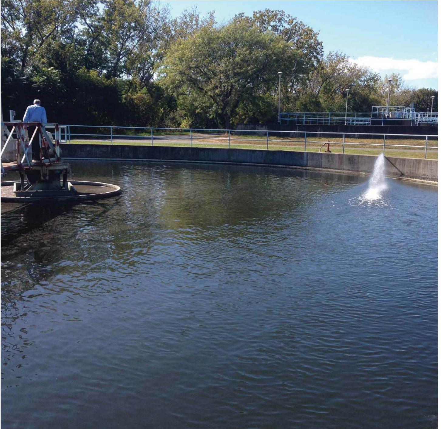
Albany County Water Purification District Water Treatment Plant. A water clarifier at the County's water treatment plant, where gravity and buoyancy remove suspended solids and other particulate matter. From here, water moves on to secondary treatment, where bacteria are used to remove organic compounds. Photo credit: WAMC
